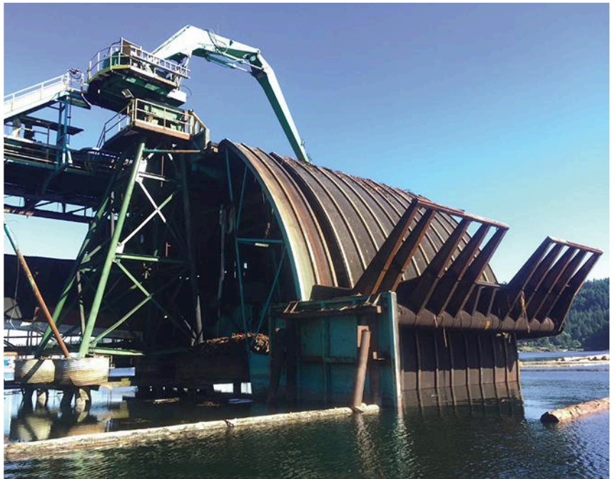
1. The arms that lift bundles of logs out of the bay and into the sawmill is operated by two 31-in.-long hydraulic cylinders.
